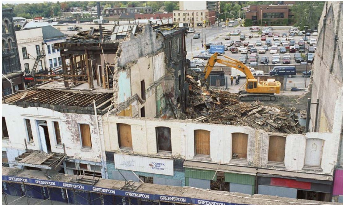
Photo 4: In 1991 London's Talbot Block was flattened to make way for private development which never came. The city ended up with the property minus its designated buildings. Photo Courtesy of the London Free Press Collection, D.B. Weldon Library, UWO.
