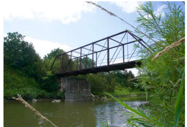
Figure 78. Bridge No. 6 spanning the Nith River at the end of Chalmers Forrest Road.
