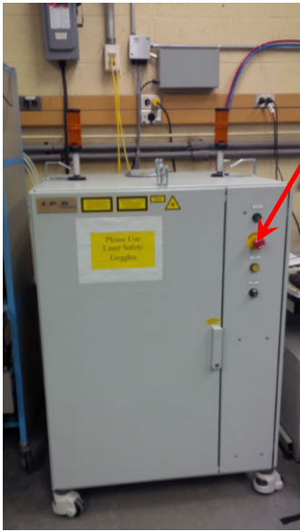
Laser Emergency Stop
