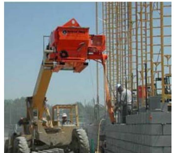
Grout delivery system
