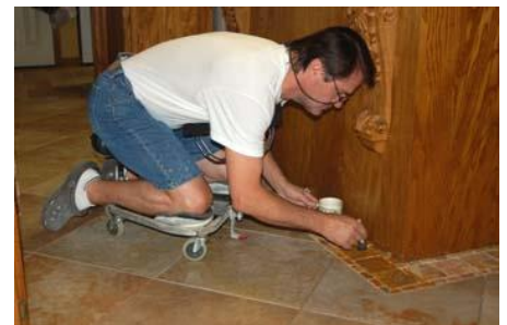
Performing detail work at floor level while positioned on a knee creeper
