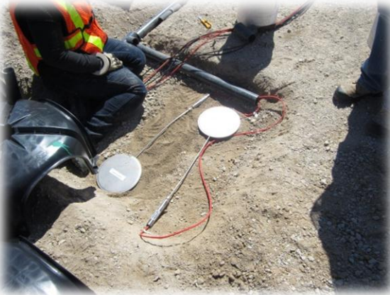
Pressure cell sensor installation on April 5, 2012 at the Milton Dufferin Quarry
