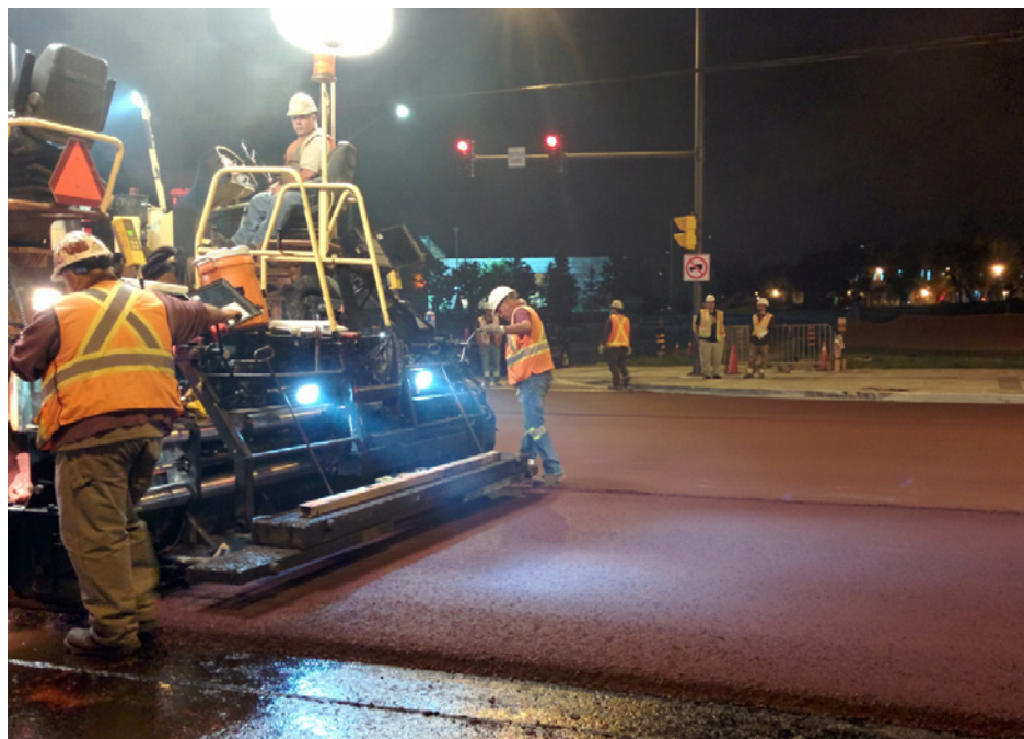
Red Asphalt paving on a section of Hwy 7 BRT Lane, York Region, August 2014
