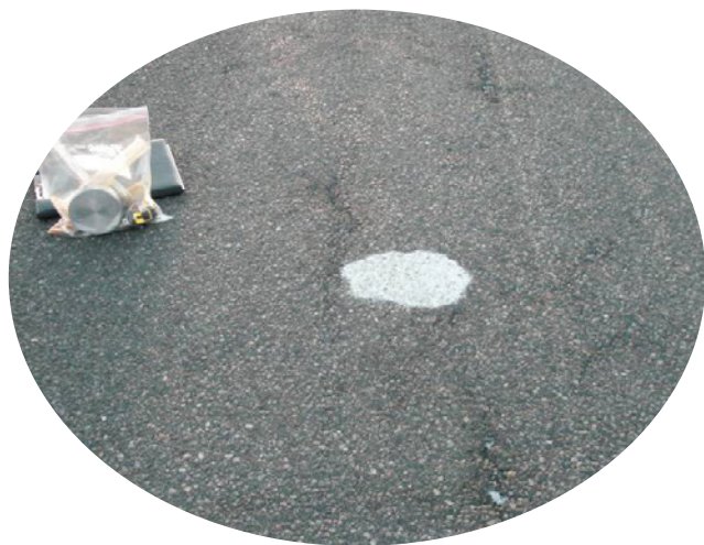
Sand patch test in area of fatigue cracking on Runway 07-25
