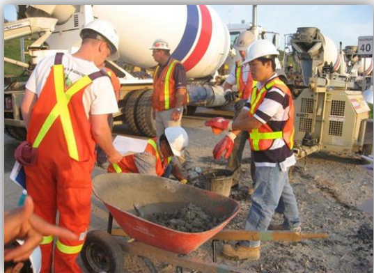
Constructing the Concrete Test Sections that contain various amounts of Recycled Concrete Aggregate
