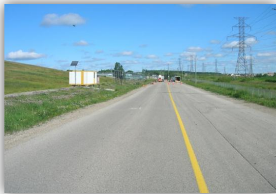
CPATT Flexible Test Sections – 8.5 years old, still performing well under heavy traffic
