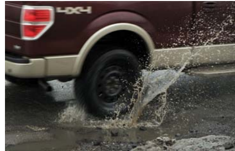
Patching up potholes, like this one on Bridge Street in Kitchener, has been a challenge for public works this winter.
