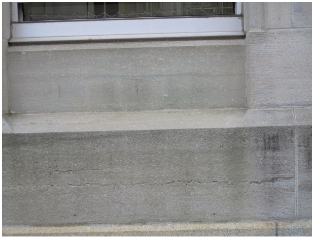
(Left) Evidence of salt damage.
