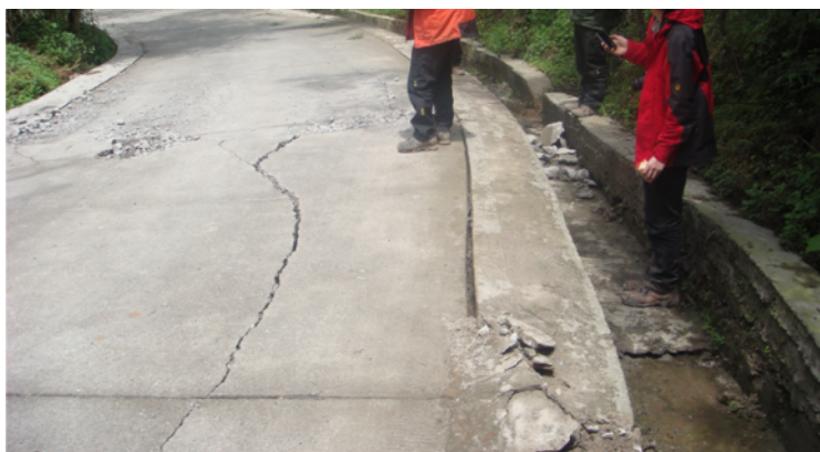
Figure 4 Road damage caused by earthquake in the southern segment of Longmenshan fault zone (LFZ). The photo was taken in Baoxing Country Daxi Town Caojia Village (E 102.80° N30.18°), Southwest China.
