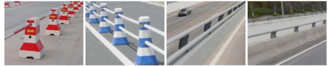
Fig. 1. Guardrails on urban roads (the lane-separating guardrails on the left and the anti-fall guardrails on the right).
