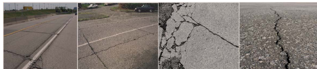
Fig. 1. Examples of pavement cracks.
