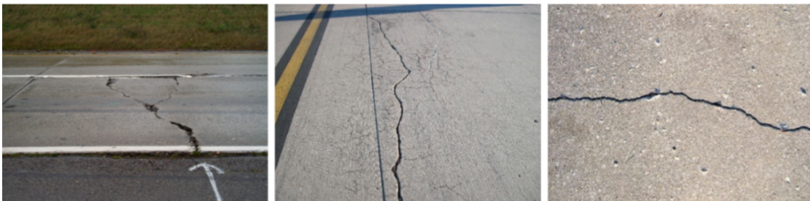
Fig. 1. Pavement cracks with different health conditions.
