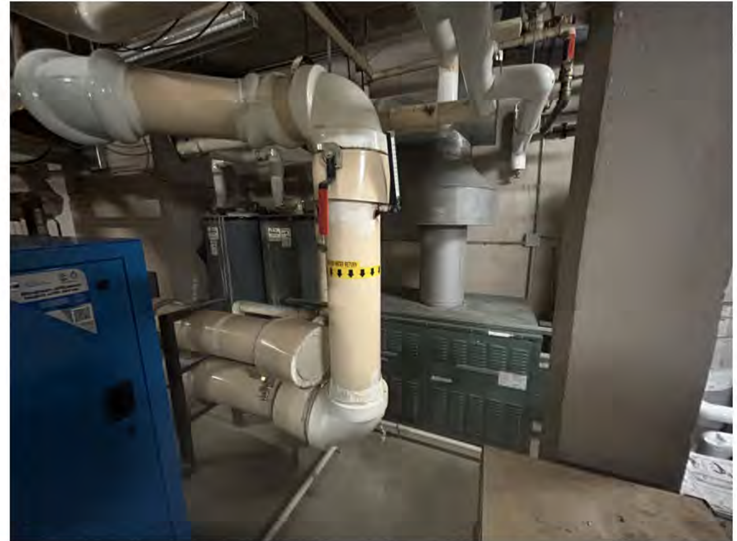
Existing domestic water tanks pictured here serving the residence washrooms. Propose replacing with three AO Smith CAHP-120 (or similar)
