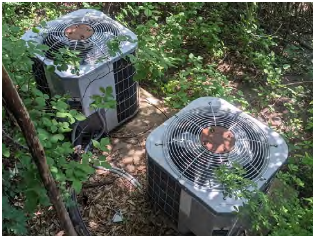
Figure 26: Cooling 1300s condensers
