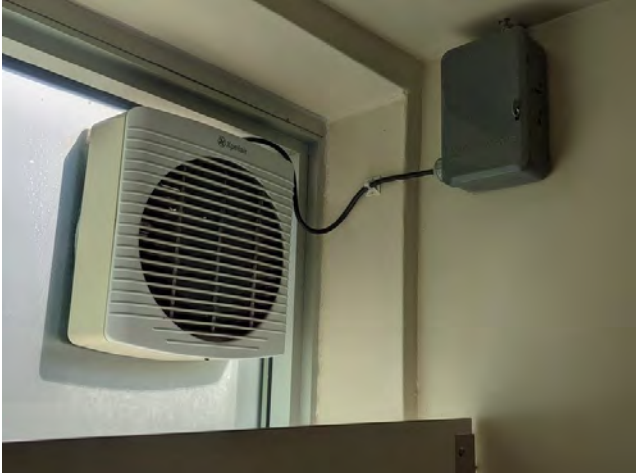
Figure 38: Exhaust fan residence
