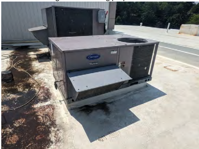
Figure 32: Cooling RTU lower atrium
