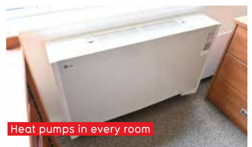
Controls for each room
