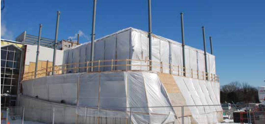
Tarps cover in the block walls that are being laid to create the archive vault that is at the heart of the 3rd floor. Winter construction has its challenges but the heaters are making it possible for the Nith Valley team to keep moving ahead.
