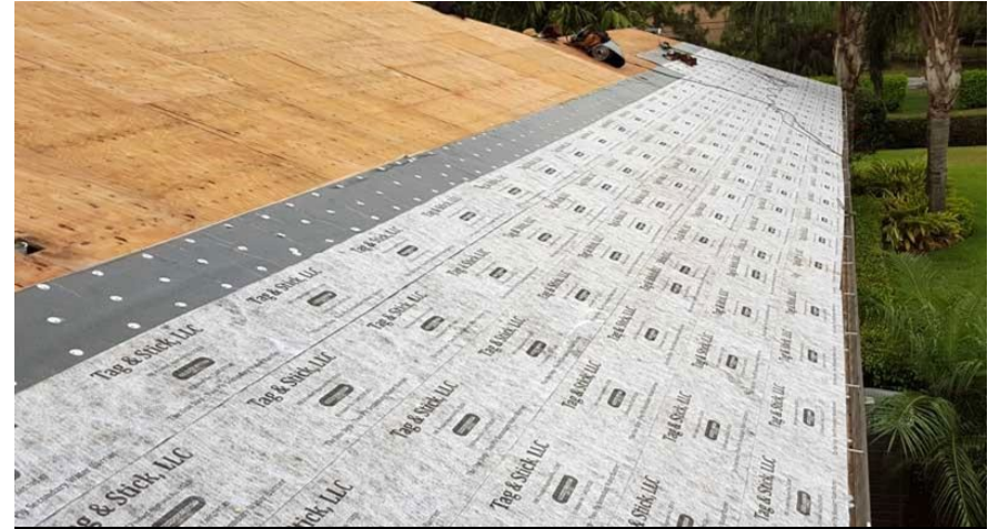
Secondary waterproofing layer
