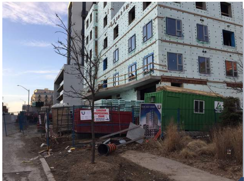
Figure 19: An example of a street tree threatened by new development (246 Lester Street)
