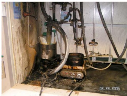
Damaged Fume Hood
