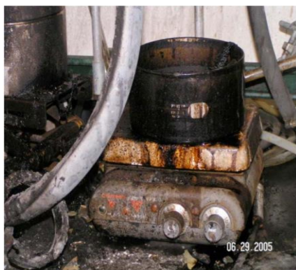
Defective Hot Plate
