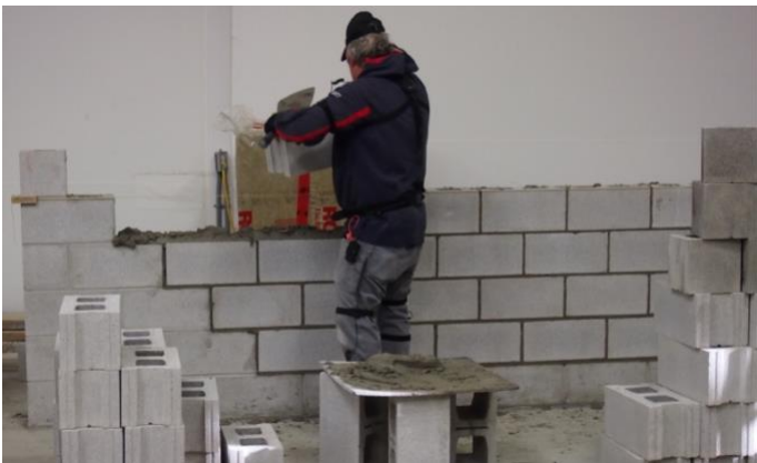
FIGURE 2. COMPLETION OF LEAD WALL BY PARTICIPANT
