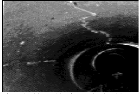
Figure 2: CCTV video image showing joint and longitudinal crack.
