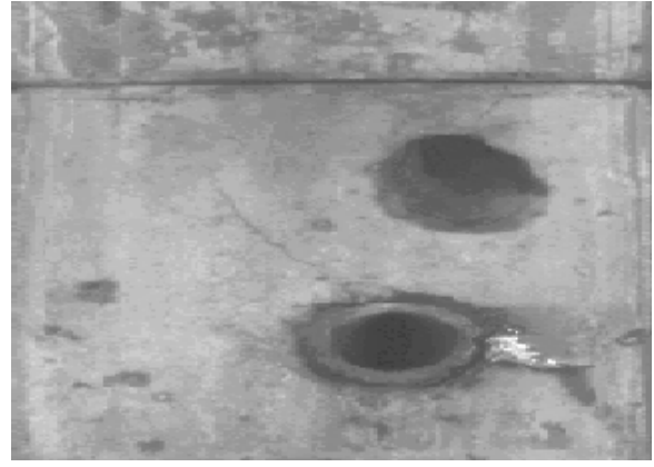
Figure 10: Pipe image showing a joint, two laterals, and minor defects.
