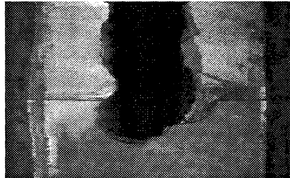
Figure 1: Underground pipe image showing a large hole, scanned by PSET (Core Corp.) in the city of Albuquerque.
