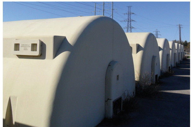
Nitrifying rotating biological contactors at the Guelph wastewater treatment plant. (Laura Sauder)
