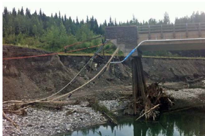
The washed out highway 66 bridge in Kananaskis Country, near Bragg Creek. Photo by Marek Stastna
