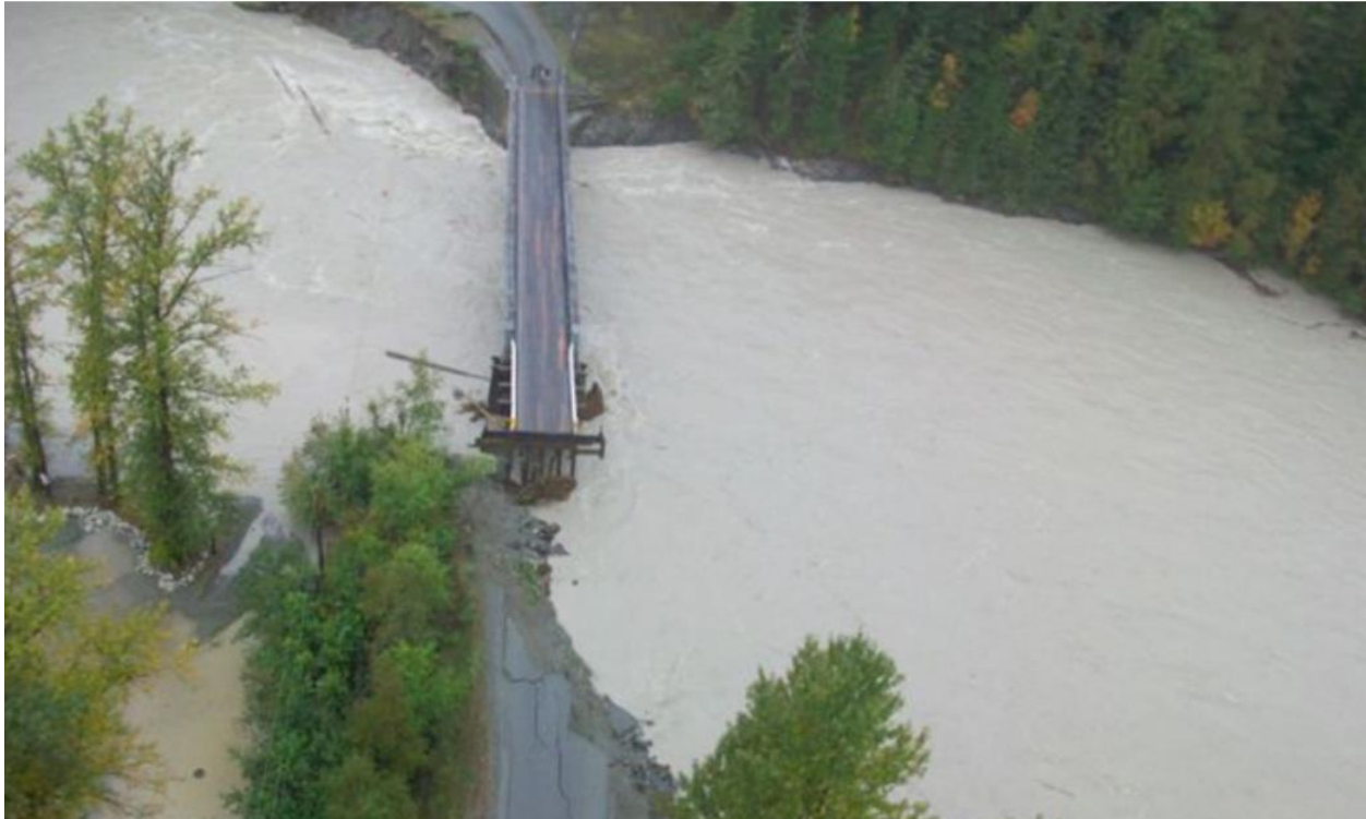
Figure 2: Highway bridge washout, Bella Coola, British Columbia in 2010 cost $45 million to repair (courtesy, B.C. Ministry of Transportation & Infrastructure).
