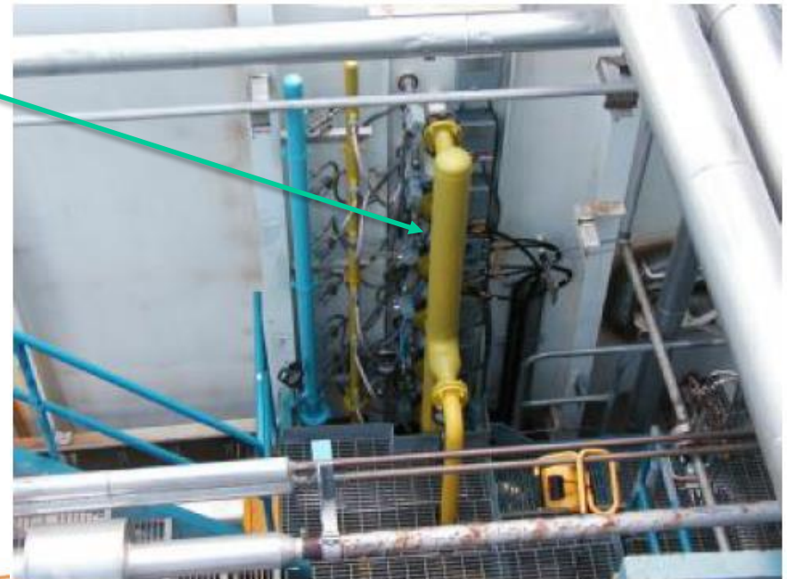
Exterior gas manifold
