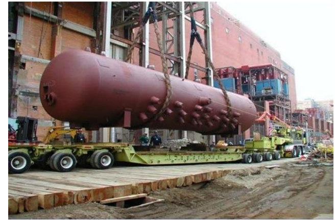
Typical Steam Drum (can be > 3" thick wall)
