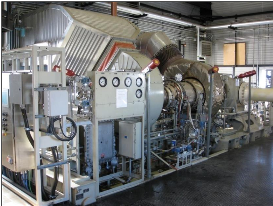
Turboden: ORC turbine / regenerator / generator
