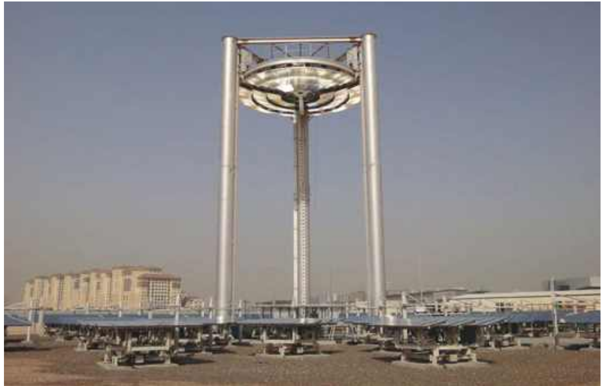
Beam-down point-focus CSP heliostat array at Masdar
